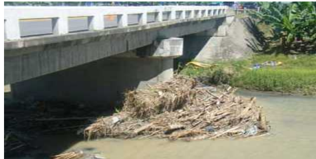
Photo 4-17 Accumulated Drift Wood and Plants around Pier
