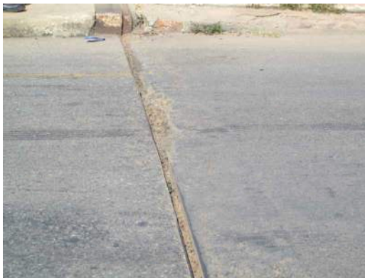
Photo 4-5 Joint is Clogged with Sand and dirt
