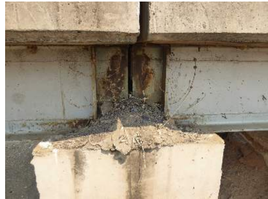
Photo 4-4 Vegetation and Soil on the Girder
