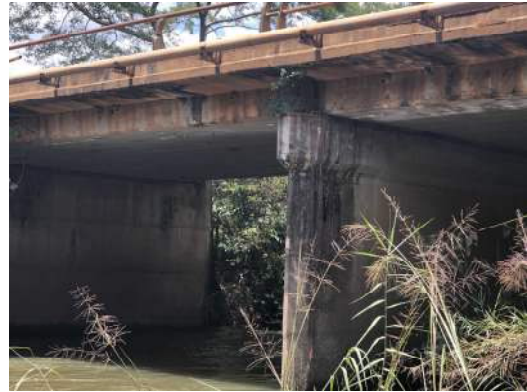
Photo 4-16 Tree Hanging Over the Girder
