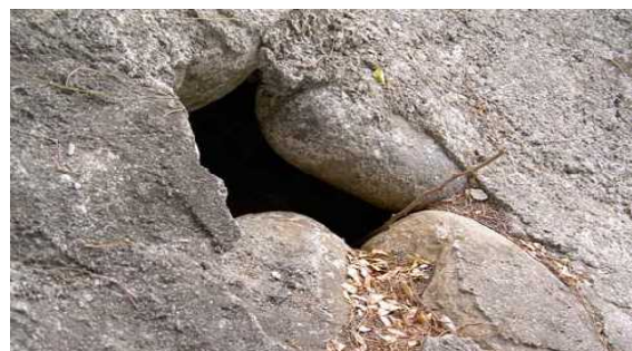
Photo 4-18 Missing Stone on Wet Masonry
