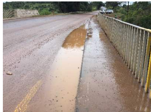
Photo 4-6 Ponding Water and Mud on the Deck
