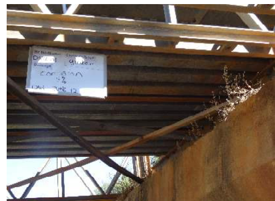
Figure 8-23 Corrosion of a Bailey Bridge
