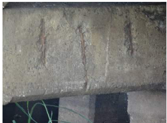
Figure 8-11 Rebar Exposure in the Girder
