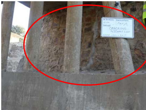
Figure 8-5 Horizontal Crack in Pier Abutment
