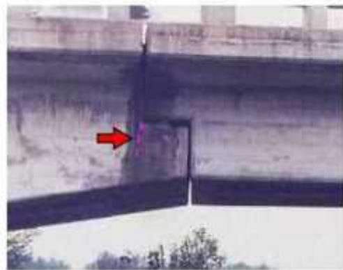
cracks in Gerber hinge
