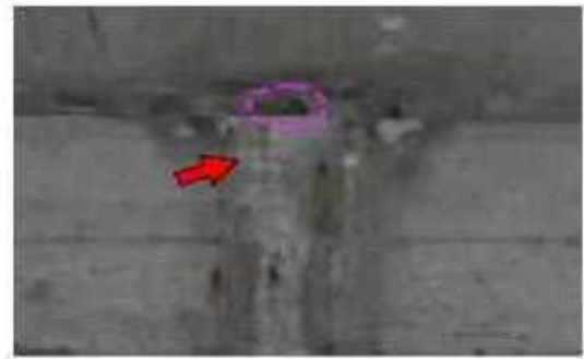
leakage from casting aperture
