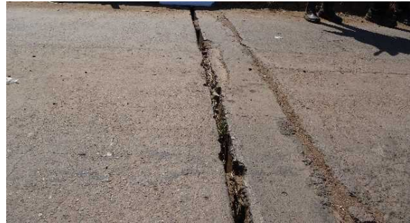
Figure 8-46 Missing Sealant (Cause of Water Leakage)
