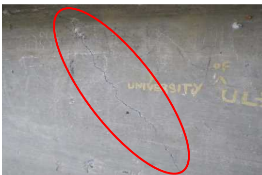
Figure 8-3 Shear Crack in a Concrete Girder
