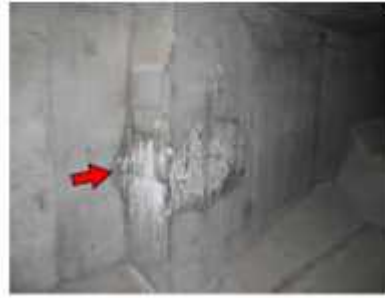
water leakage from the projection of fixed web
