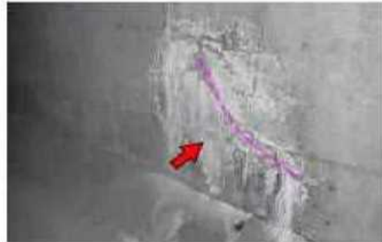
leakage along the PC steel
