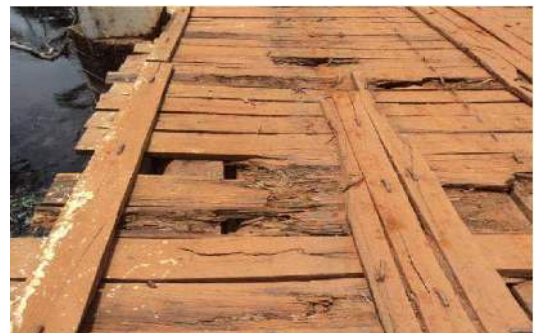
Figure 8-19 Decay of Timber Deck Slab
