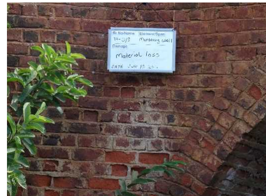
Figure 8-22 Material loss of an Arch Bridge
