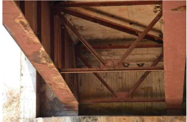
Figure 8-14 Corrosion of Steel Member
