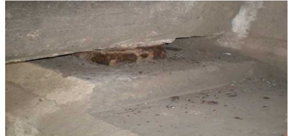
Figure 8-26 Corrosion of Steel Bearing
