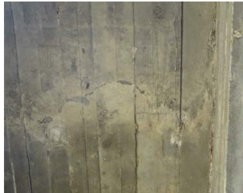
Figure 8-10 Delamination in Deck Slab
