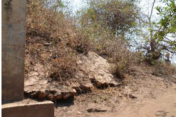
Figure 8-35 Cracking in Slope Protection
