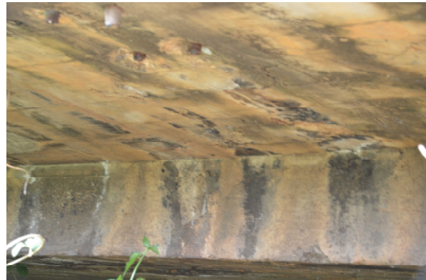
Figure 8-13 Water Leakage from Some Holes for the Anchor Bolt
