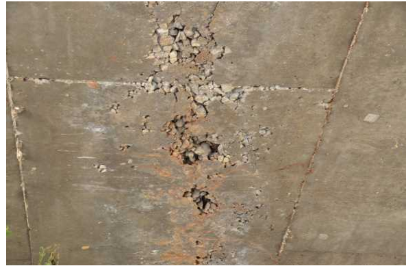
Figure 8-12 Honeycomb in Deck Slab
