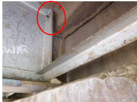
Figure 8-17 Loose Connection of Steel Member
