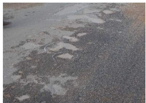
Figure 8-53 Ravelling of Asphalt Surface
