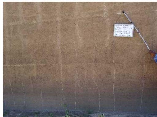
Figure 8-7 Vertical Cracking by Differential Settlement
