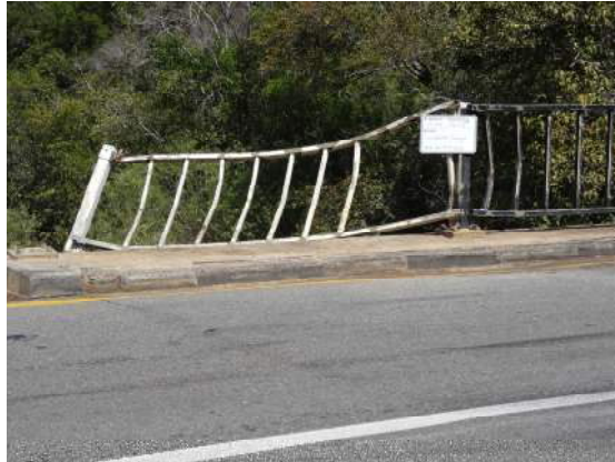
Figure 8-50 Accidental Damage of Railing
