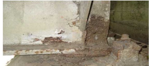
Figure 8-27 Abnormal Displacement at a Support
