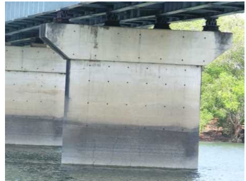
Figure 8-30 Tilt of Pier
