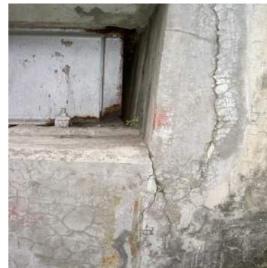
Figure 8-32 Settlement of Abutment
