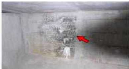
water stain along PC steel
