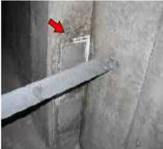
water stain on the postcasted area
