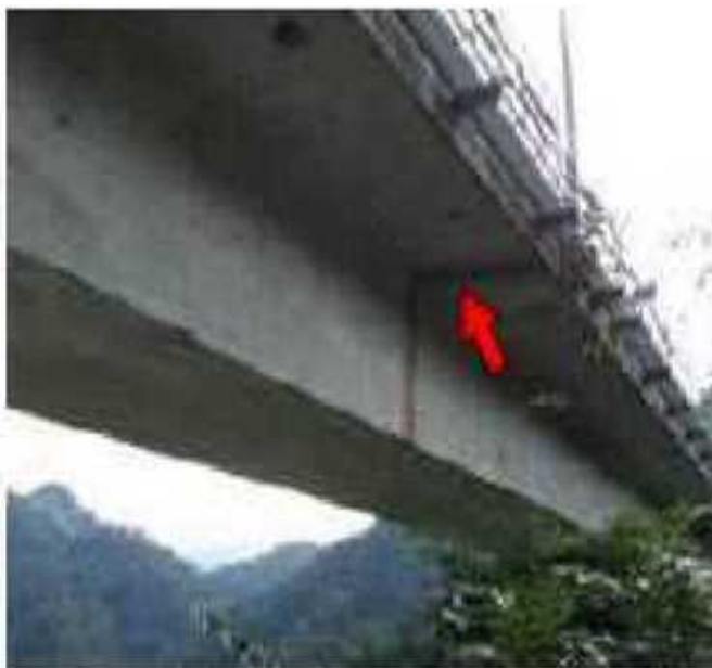
Water leakage from outer surface of box girder
