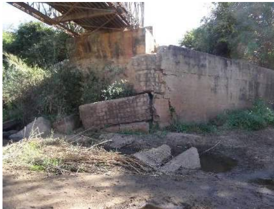
Figure 8-36 Slope Protection Erosion
