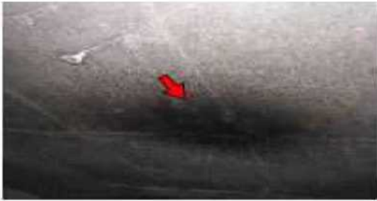
Water stains around central parts
