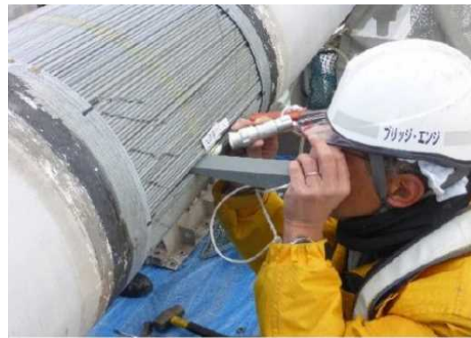
Figure 3-4-4 Internal main cable inspection (cable wires were wedged)
