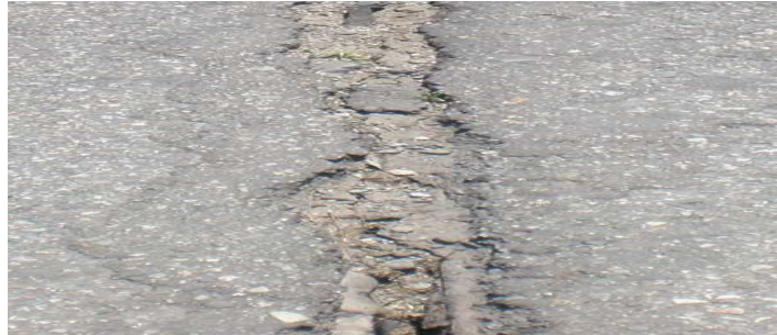
Figure 8-43 Water leakage Due to Deteriorated Rubber Sealant
