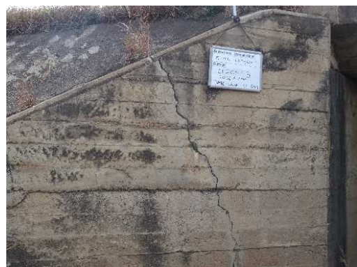
Figure 8-8 Crack in Wing Wall
