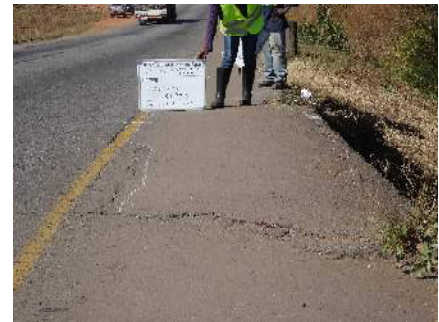
Figure 8-52 Cracking of Asphalt Surface
