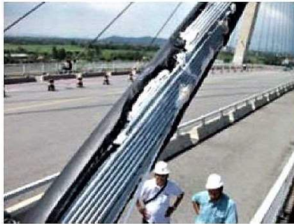
Figure 2-7-15 cable fracture conditions
