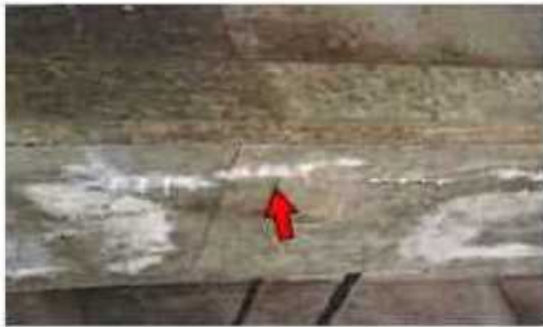
leakage from underneath the main girder
