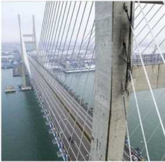
Figure 2-7-12 Conditions of stay-cable fracture
