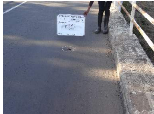
Figure 8-51 Potholes of Asphalt Surface
