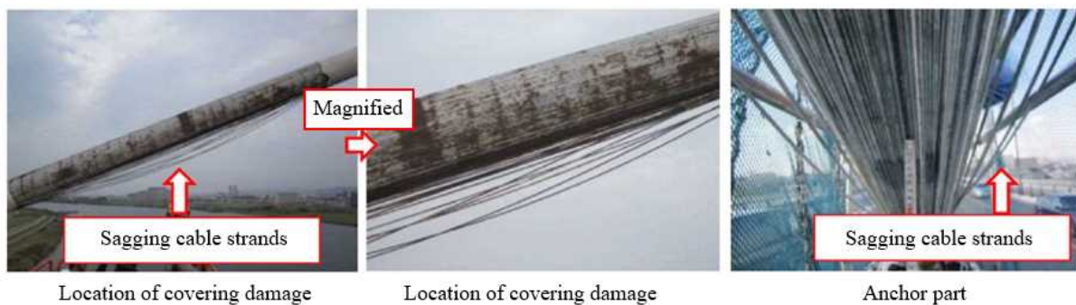
Figure 2-7-8 Example of partial cable fracture caused by corrosion
