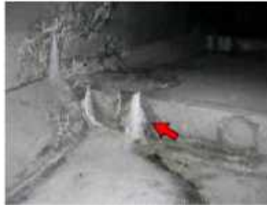
water leakage from the projection of lower floor slab
