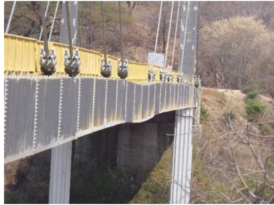
Figure 8-16 Deformation of Steel Member
