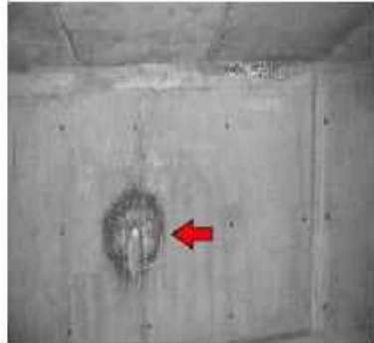
water stain on the postcasted P-con
