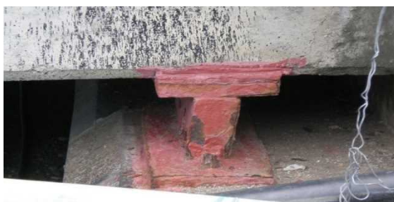
Figure 8-28 Paint Deterioration of Bearing
