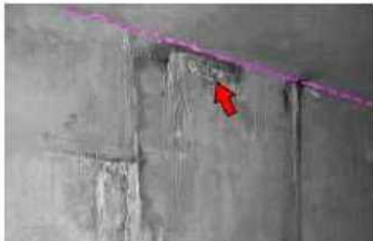
leakage from joints
