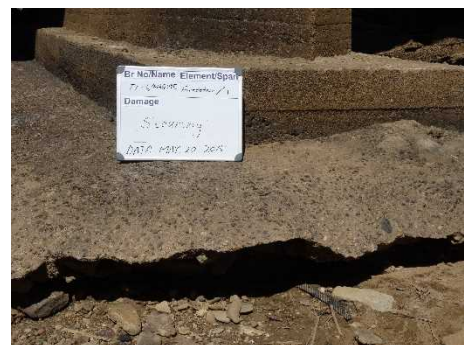
Figure 8-33 Scouring at Abutment
