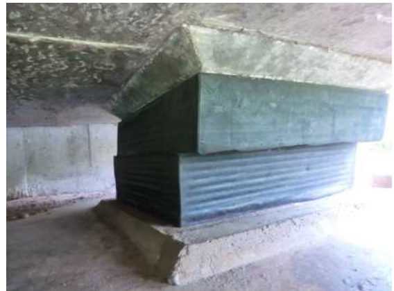
Figure 8-25 Abnormal Displacement of Bearing
