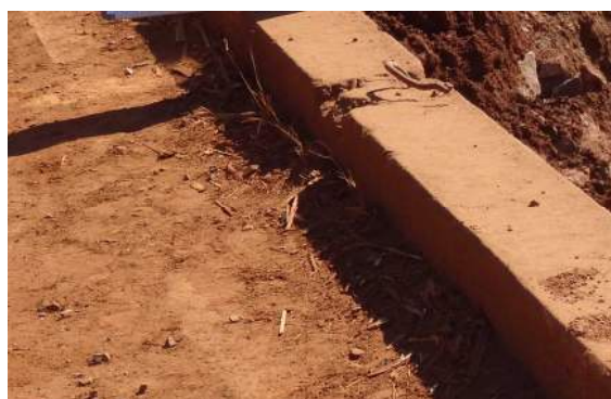
Figure 8-42 Cracking at Kerb
