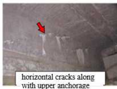
Horizontal cracks along with PC steel
