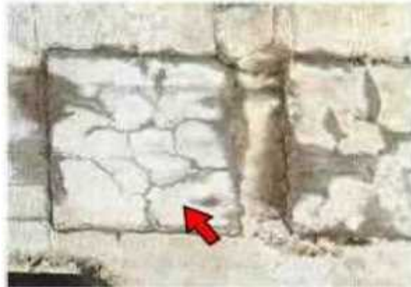
cracks in the post-filling concrete
