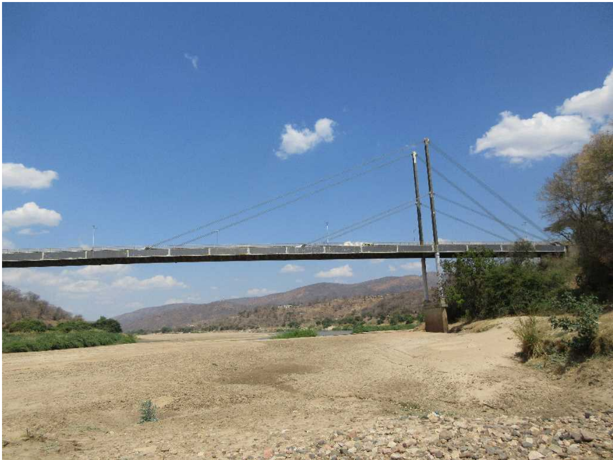
Figure 2-7-7 sagging of deck slab in Luangwa Bridge
