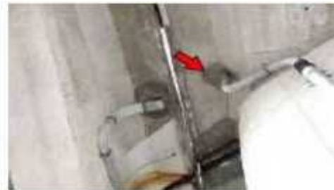
water stains around the drainage
