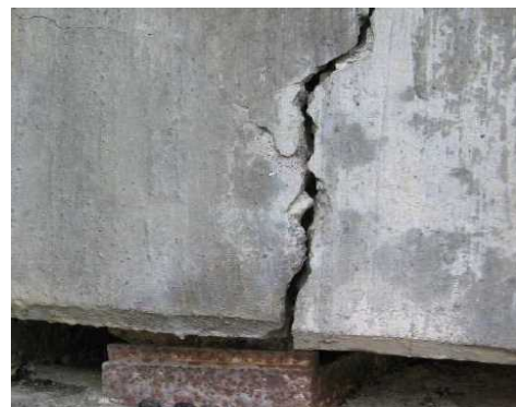
Figure 8-4 Shear Crack near the Bearing
