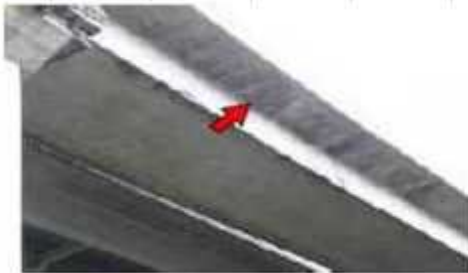
water stains shaped like worm crawling, perpendicular to the bridge axis
