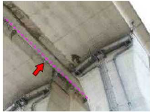
leakage from construction joints
