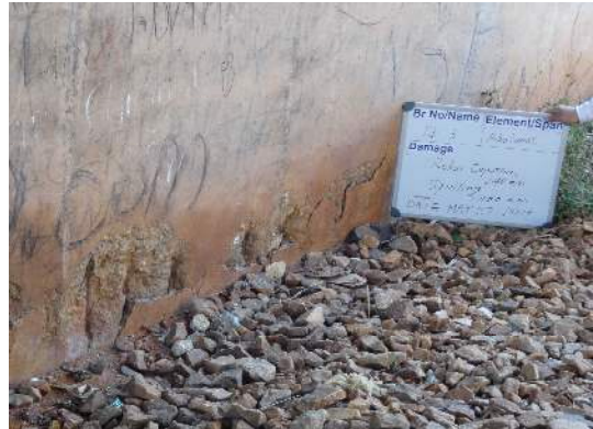
Figure 8-9 Spalling on Abutment
