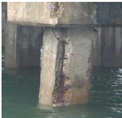
Figure 8-31 Tilt of Pier Due to Collision
