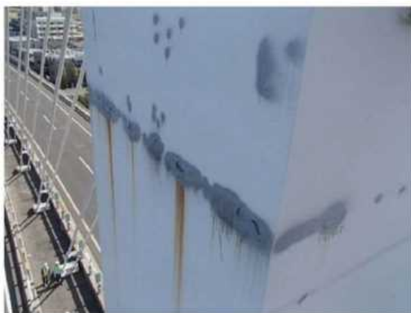
Corrosion at joint (metal touch structure)
