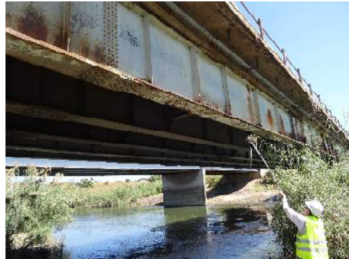
Figure 8-18 Paint Peel Off of Steel Member
