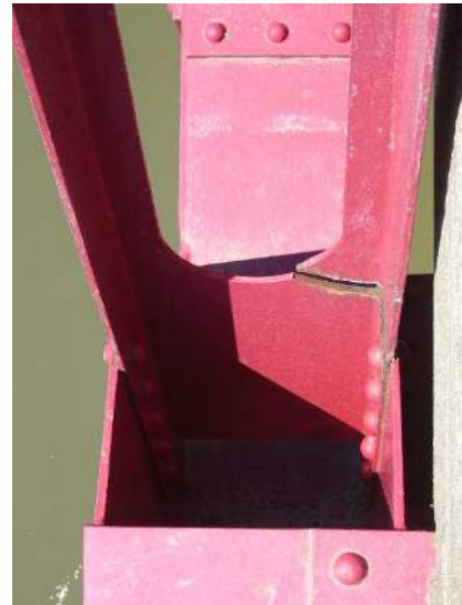
Figure 8-15 Cracking of Steel Member
