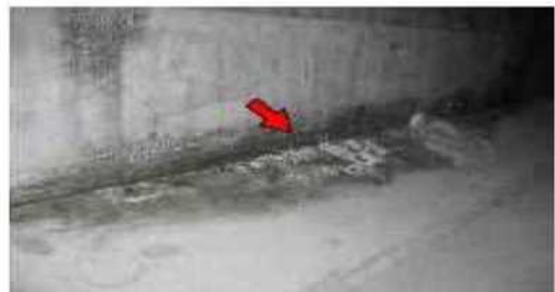
water stains around the lower floor slab haunches
