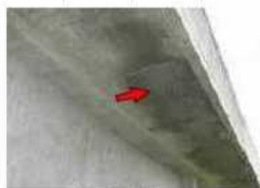
streaked water stains
