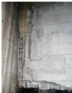
damage to the girder end
