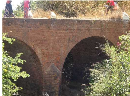
Figure 8-21 Fretting/Abrasion of an Arch Bridge
