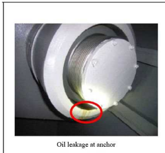
Figure 2-7-16 Example of deterioration in tower side stay cable anchor
