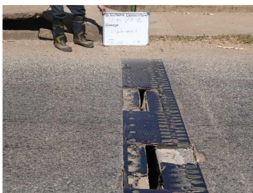
Figure 8-41 Displacement of Cover Plates
