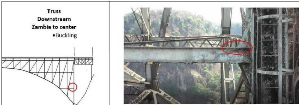
Photo 10-16 Buckling of Steel Member
