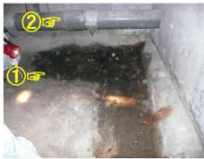
water leakage found in the girder
