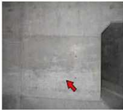
cracks in the cross girder
