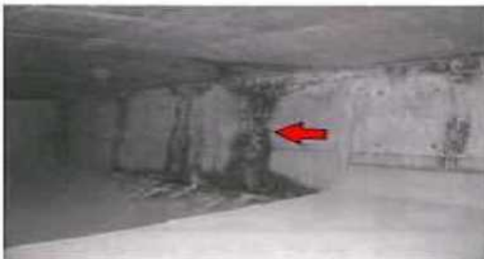
vertical water stain on the inner surface
