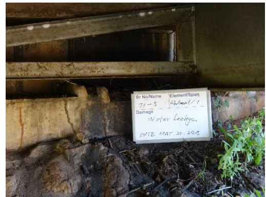
Figure 8-38 Water leakage from Expansion Joint
