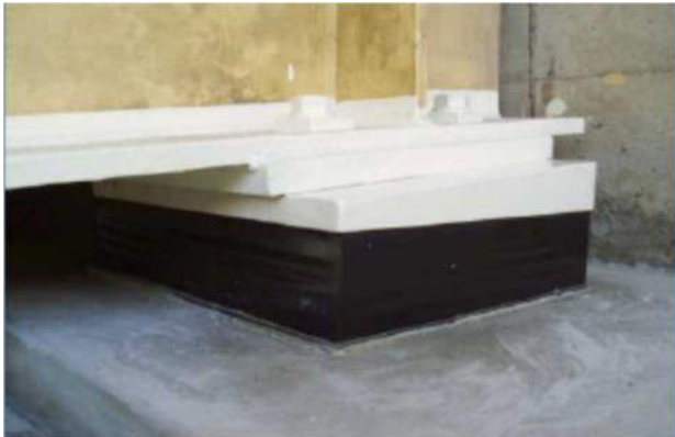
Photo 8-1 Sample of Replaced Bearing
