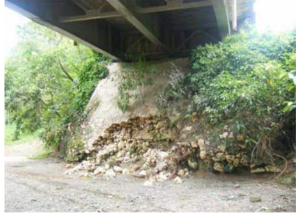
Photo 9-1 Broken Slope Protection
