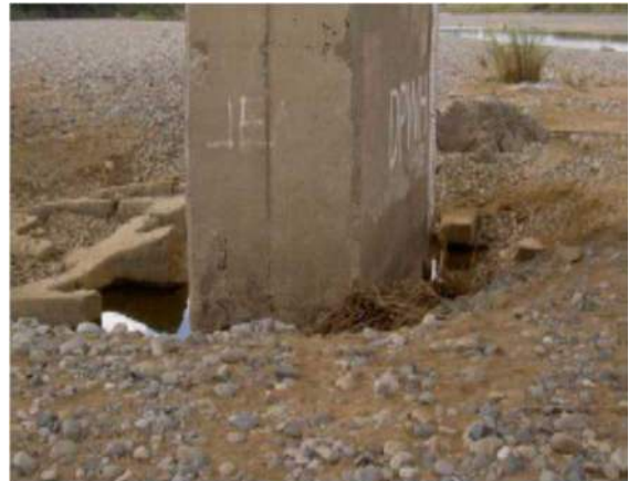
Photo 9-2 Local Scouring around Pier
