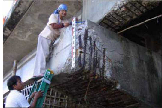
Photo 6-1 Damaged Pier for Repair by Recasting
