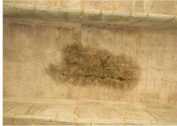
Photo 3-2 Severely Damaged Deck Slab
