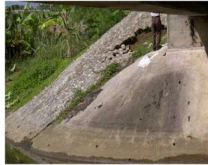
Photo 9-3 Damaged Slope Protection
