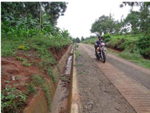
Inappropriate design of side drain
