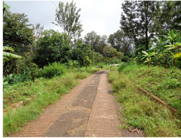
Figure 2-8: Example of poorly maintained concrete strip road
