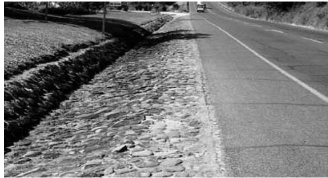
Figure 5-5: Undesirable drain design
