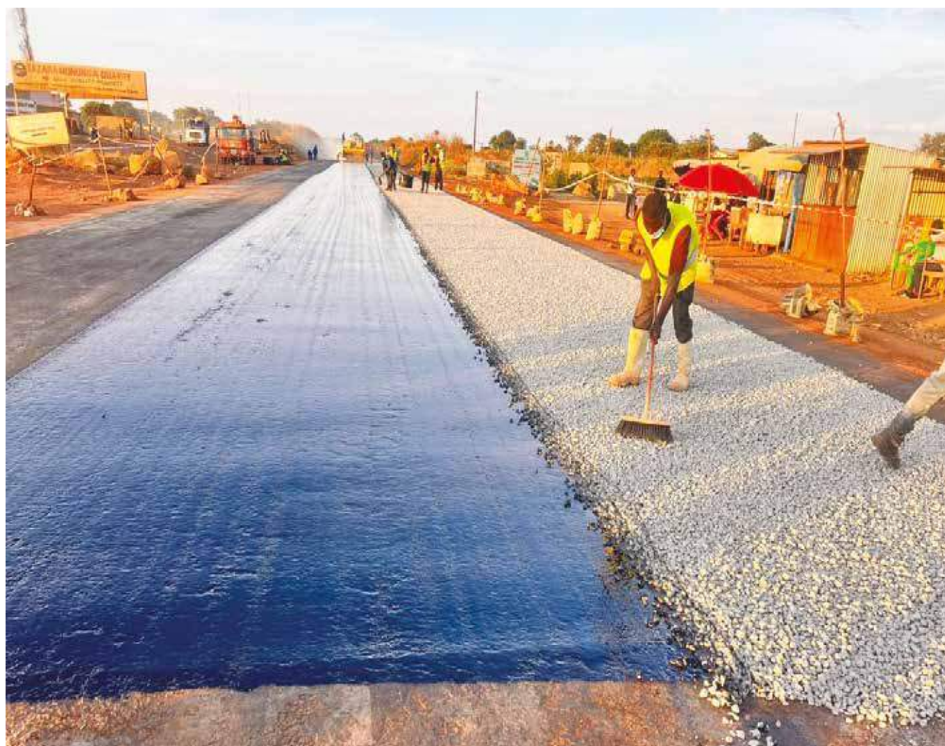
Figure 3.7: Reconstruction works on the damaged section of the Great North Road from Lukulu Bridge
