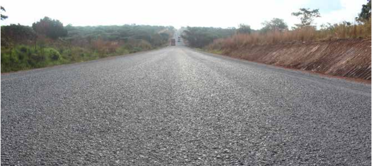
Figure 3.6: Holding maintenance works on the Great North Road between Serenje to Chinsali
