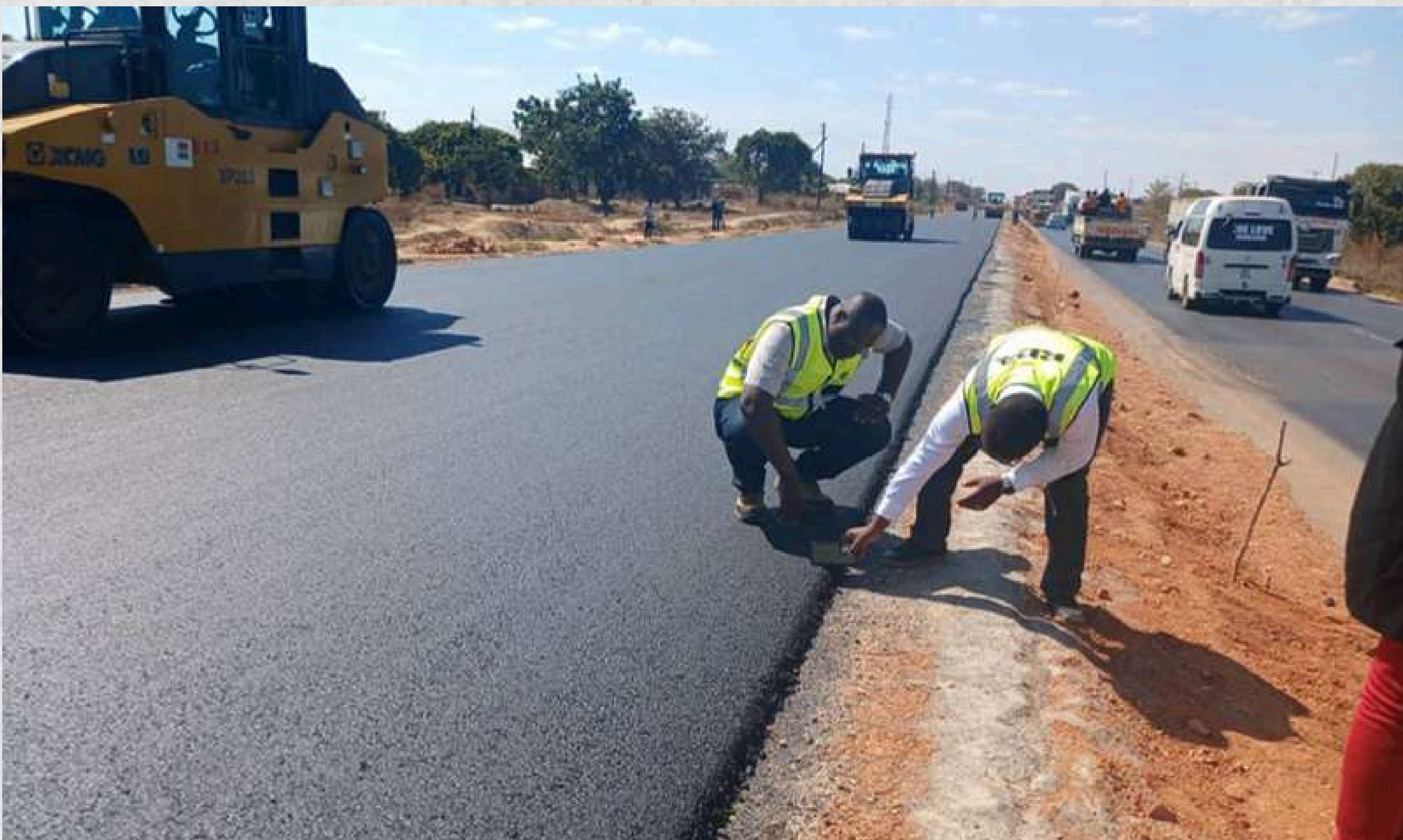
RDA Chief Communications and Corporate Affairs Manager, Anthony Mulowa (left) with RDA Senior Engineer for Public Private Partnership (PPP) Implementation, Eng. Kakoma Kalengo during a media tour of construction works on the Lusaka–Ndola Dual Carriageway.
