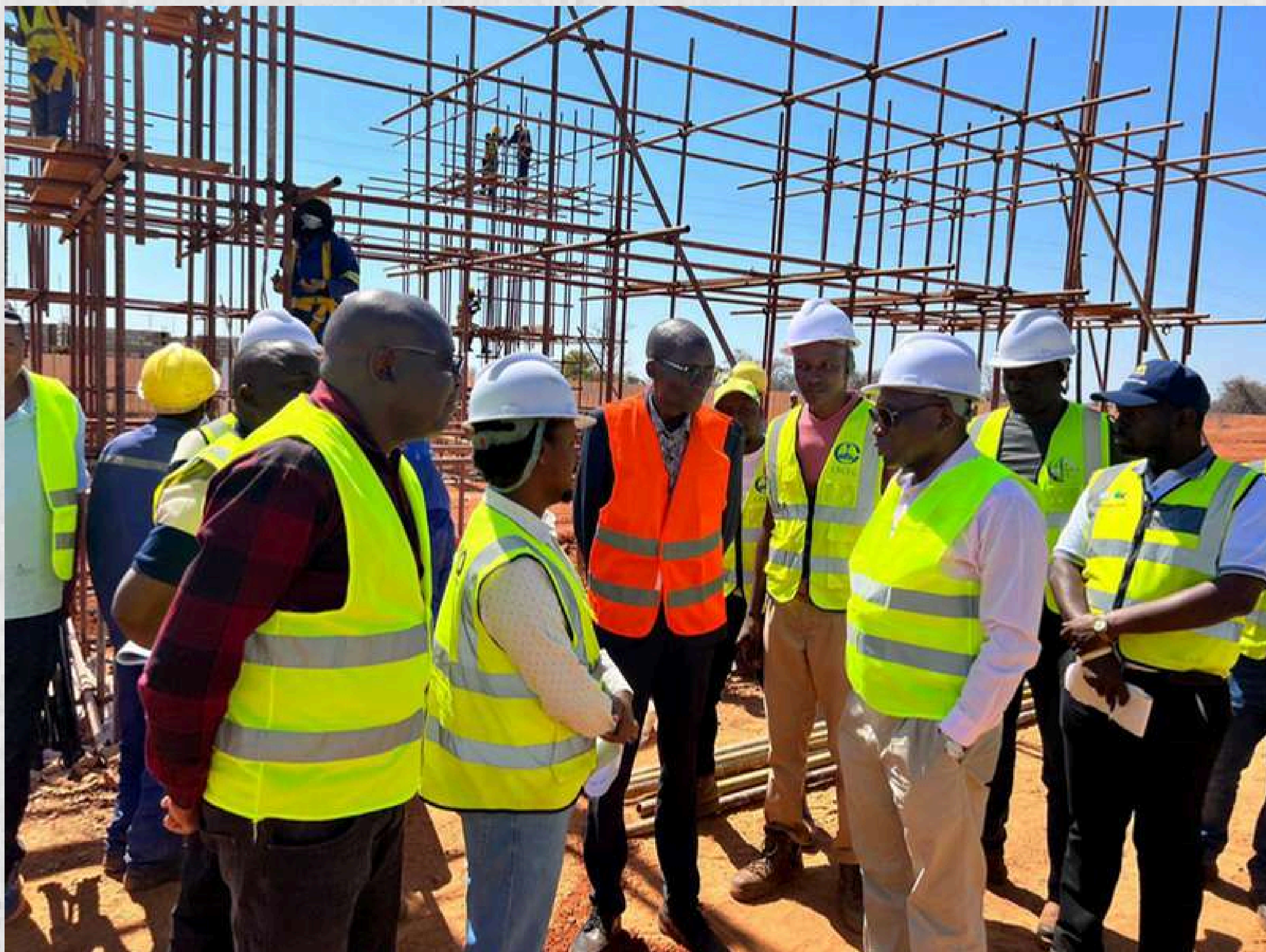
Infrastructure, Housing and Urban Development, Hon. Eng. Charles L. Milupi during the inspection of construction works of the Mazabuka Toll Plaza along the Kafue-Mazabuka Road.
