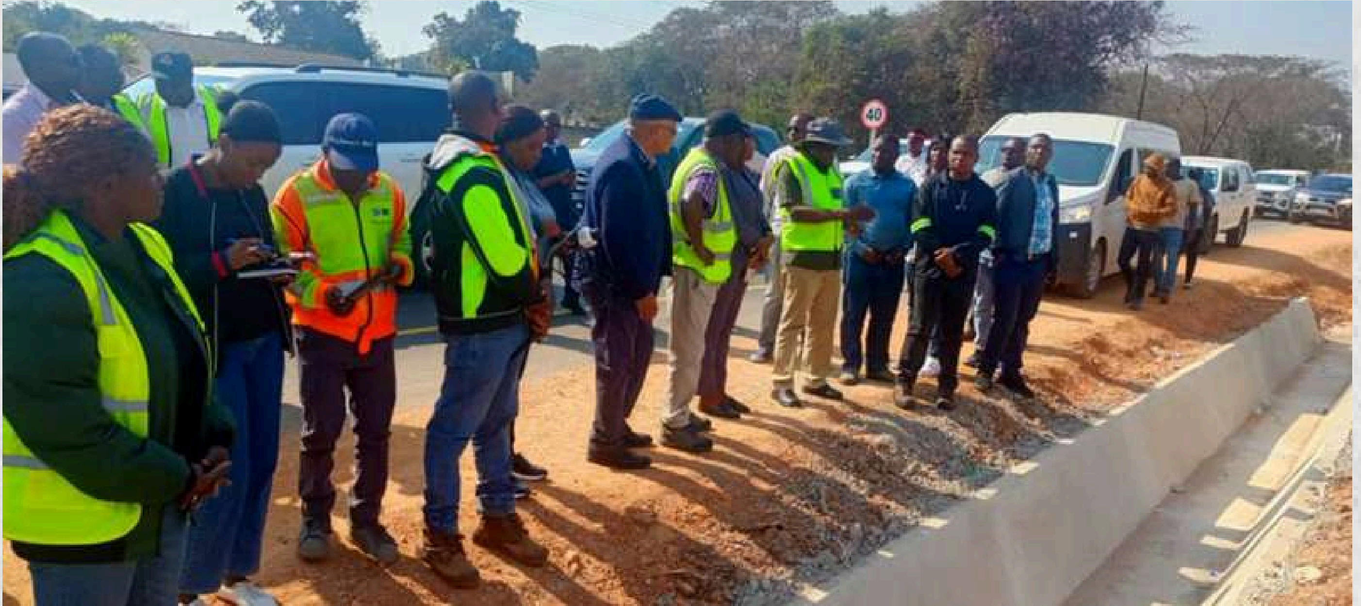
Infrastructure, Housing, and Urban Development Minister, Hon. Eng. Charles Lubasi Milupi inspecting works on the Ndola-Sakania-Mufulira Road on the Copperbelt Province.
