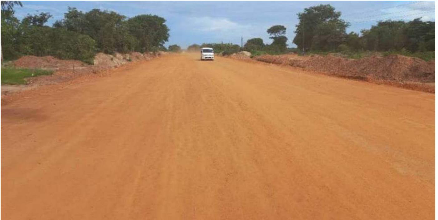
Lusaka-Mongu Road works from Tateyoyo Gate to Katunda/Lukulu Junction in Western Province.
