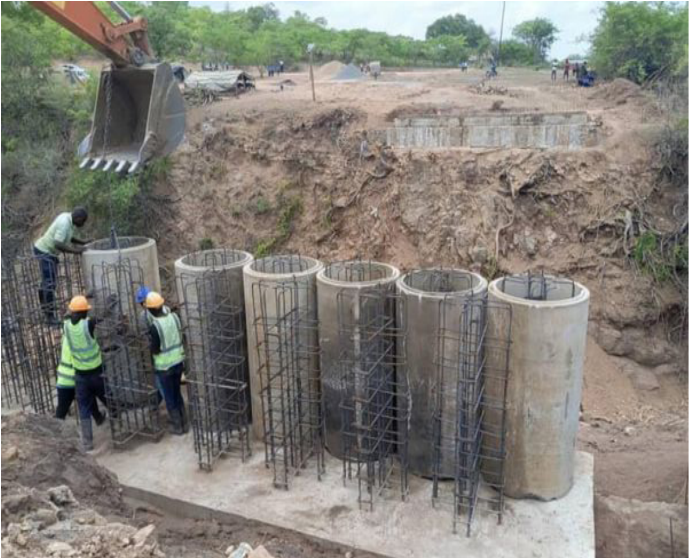
Construction of Lusangazi Bailey Bridge on the Petauke-Ukwimi Road in the Lusangazi District of Eastern Province.
