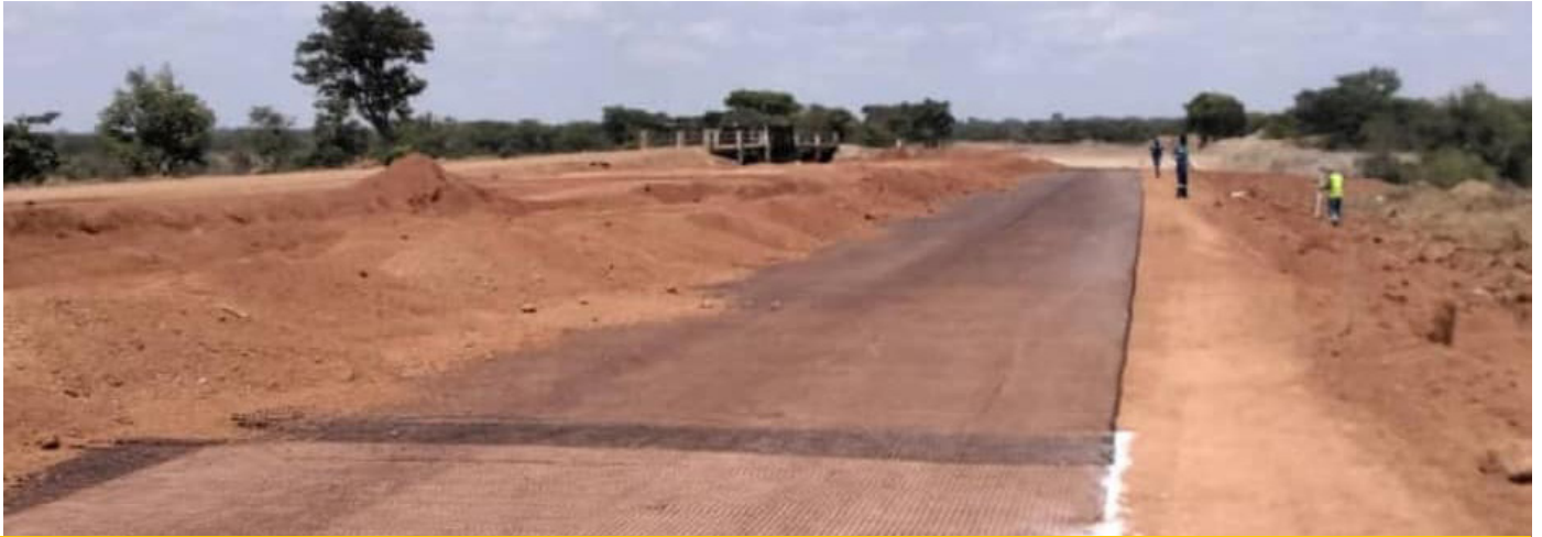
Construction works of the Kasomeno-Mwenda Road and Bridge Project in Luapula Province under the Public Private Partnership (PPP) Financing Model.
