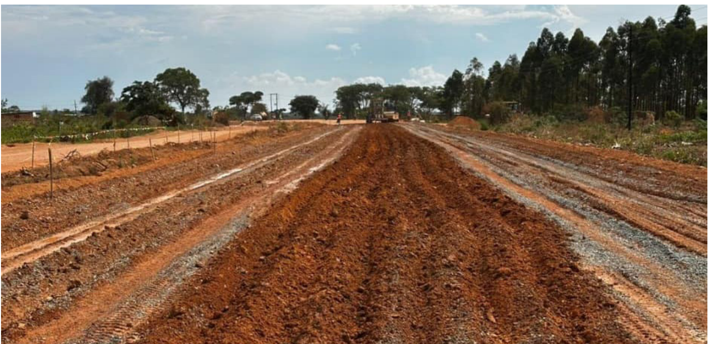
Progress on earthworks between Mitengo, about 3 kilometres from Levy Mwanawasa Stadium Roundabout and Sakania Border at kilometre 17.
