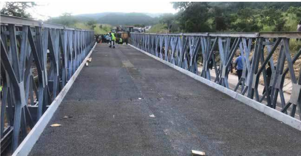
Figure 10: The Acrow Bridge which was mounted as a temporary measure at Ngozi Culvert
