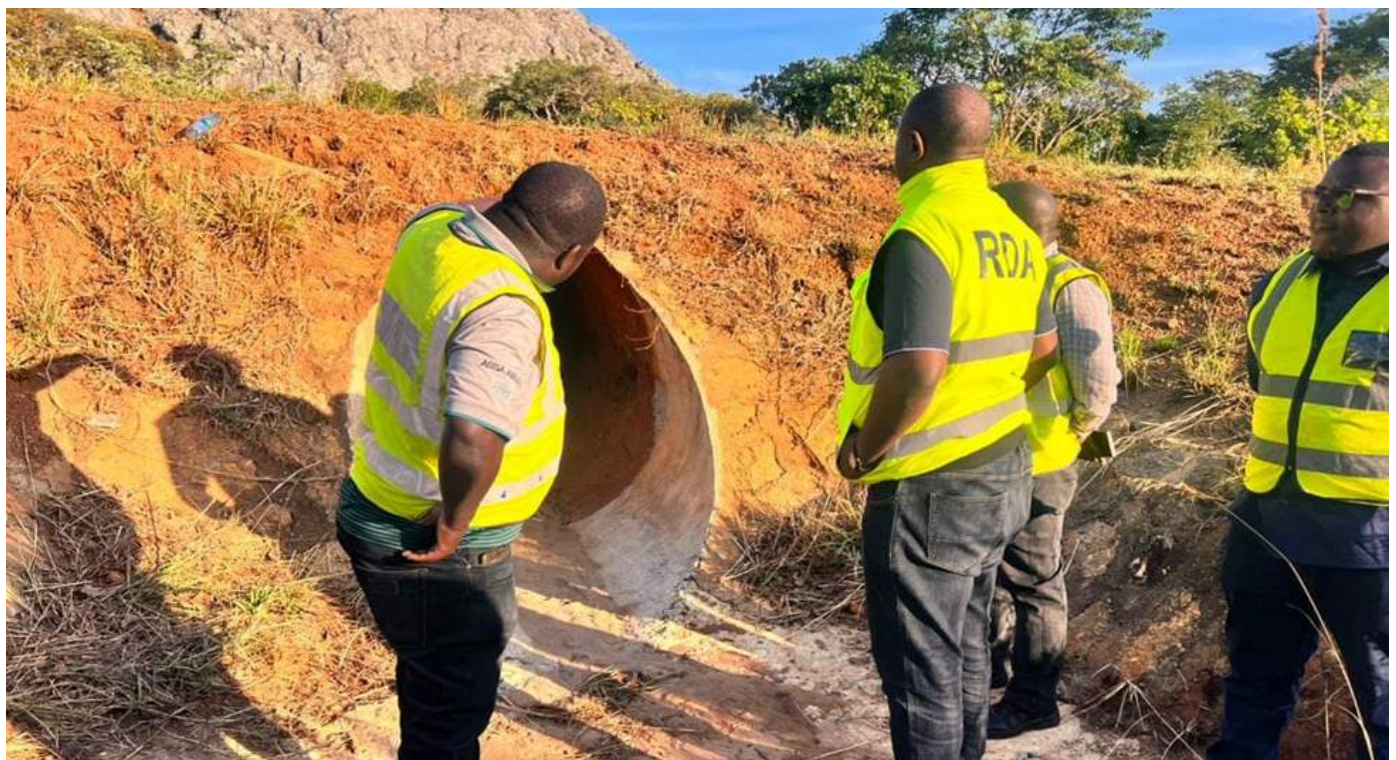
RDA Acting Director Communications and Corporate Affairs, Mr. Anthony Mulowa (middle) with Muchinga Regional Manager, Eng. Peter Sinkonde (far left) inspecting a vandalized culvert on the Great North Road.
