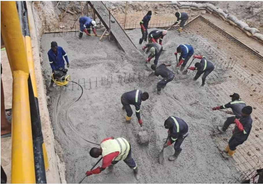
Construction works at the Gibson Chimfwembe and Lulamba box culverts in Chingola District.
