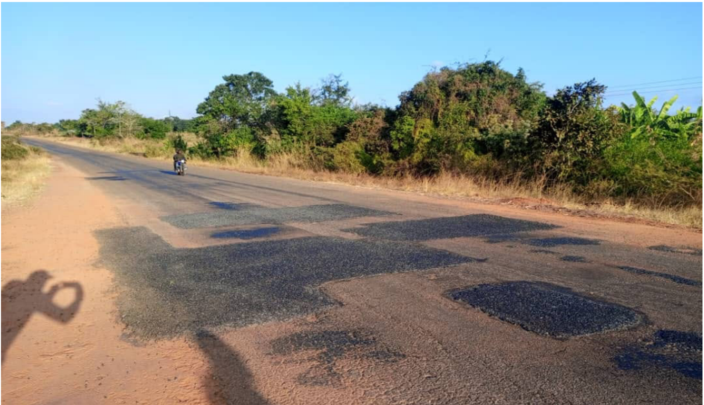
Patched section of the Chiptata-Mfuwe Road.
