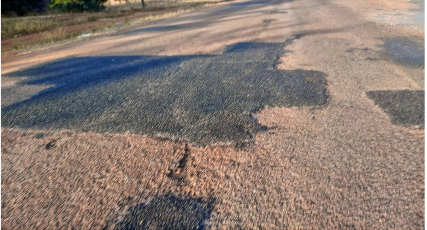
Patched section of the Chipata-Mfuwe Road.
