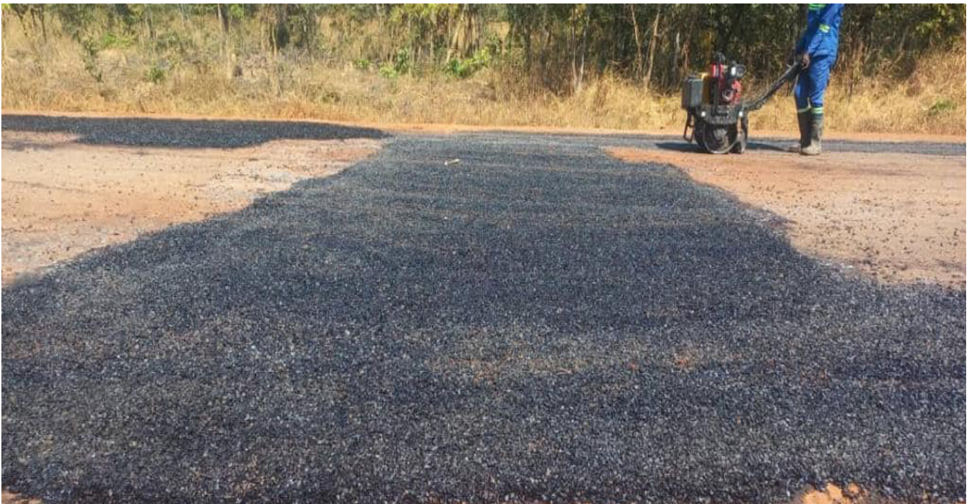
The patched section of the Luansobe to Mpongwe Road.
