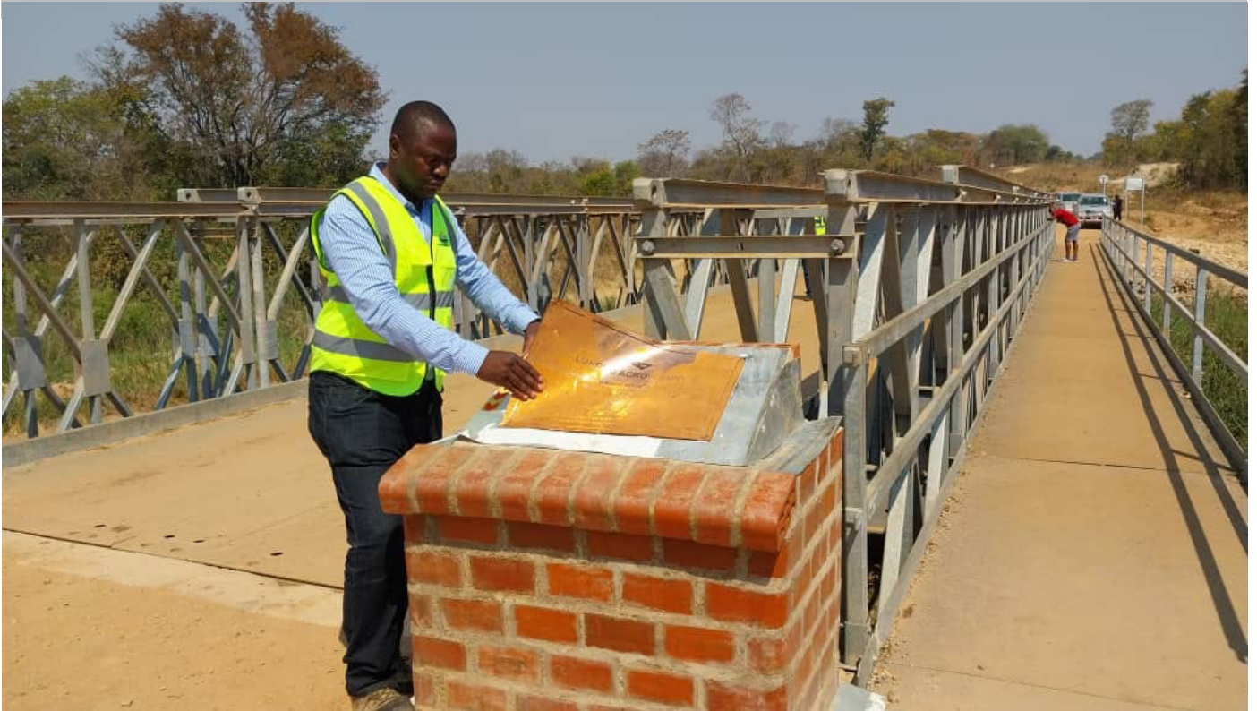
RDA Acting Director Communications and Corporate Affairs, Anthony Mulowa inspecting the vandalized plaque at Lunchu ACROW Bridge.
