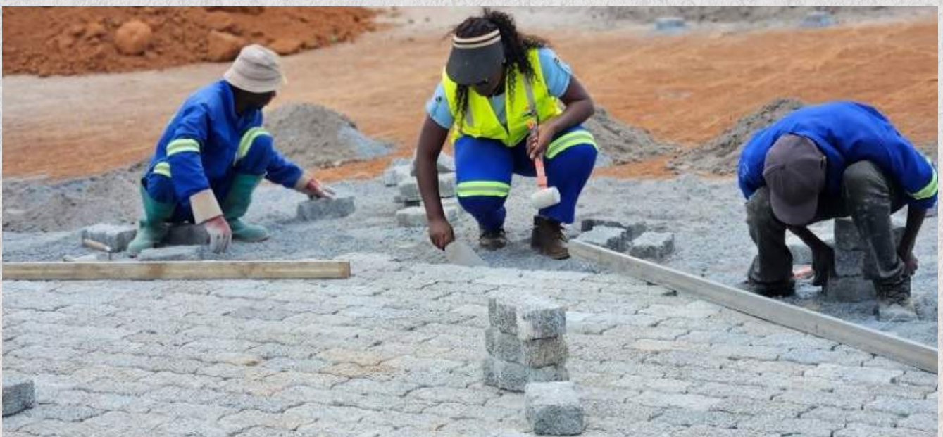
Eng. Faith Chisata (middle) on site paving the driveway at Sabina Toll Plaza along M16 Road on the Copperbelt.
