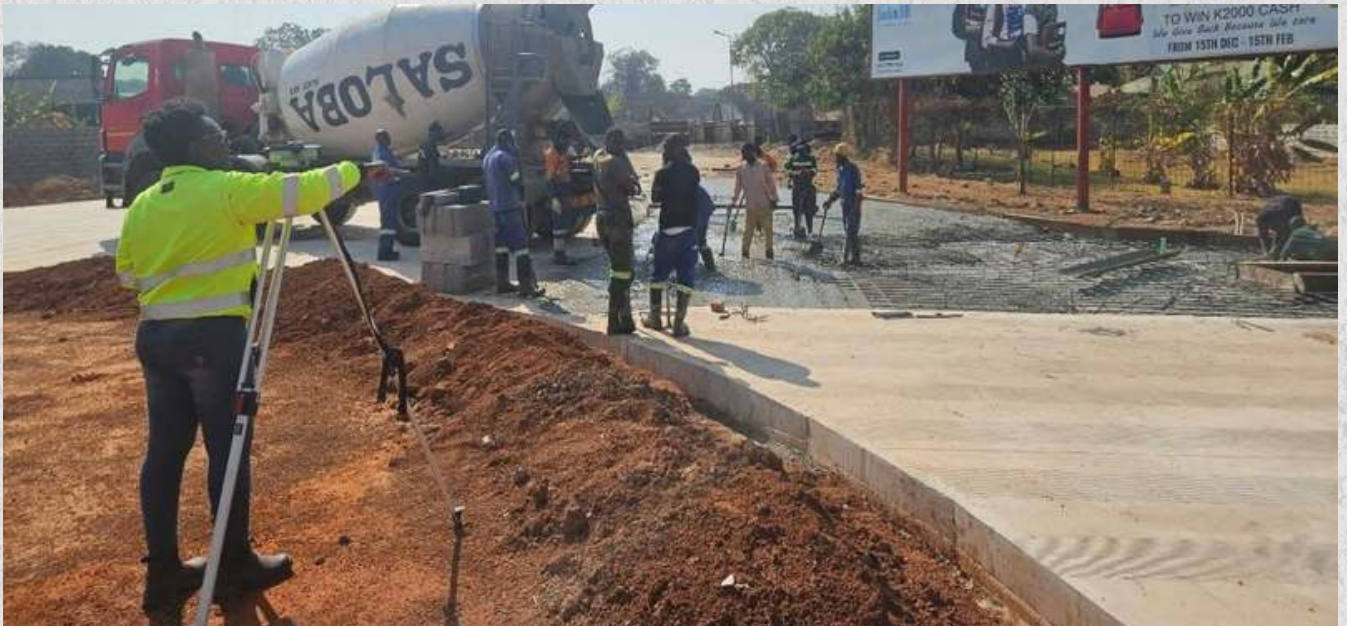
Eng. Faith Chisata on site: Construction of Chatulinga Roundabout in Mufulira on the M005 Road.
