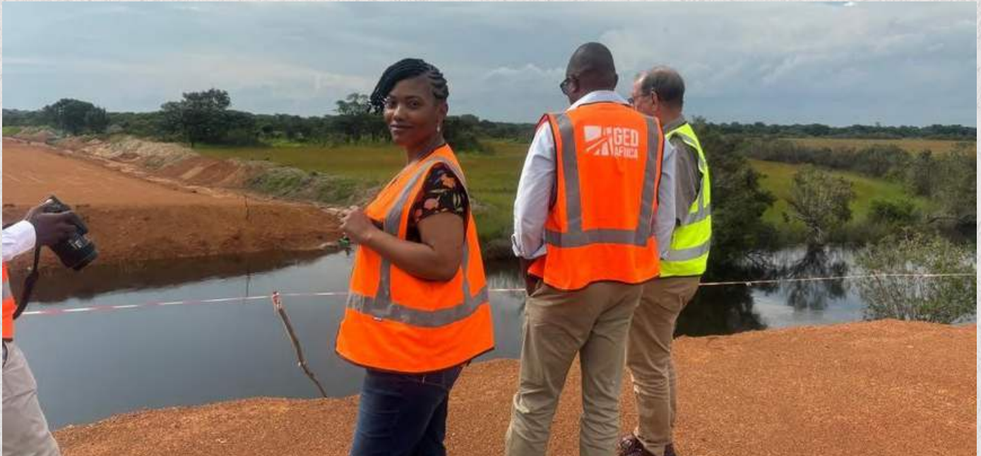
Embankment fill at Luongo Bridge under the Kasomeno Mwenda PPP Road Project where Eng. Namukonde was checking the progress made on the construction of the Luongo Bridge.
