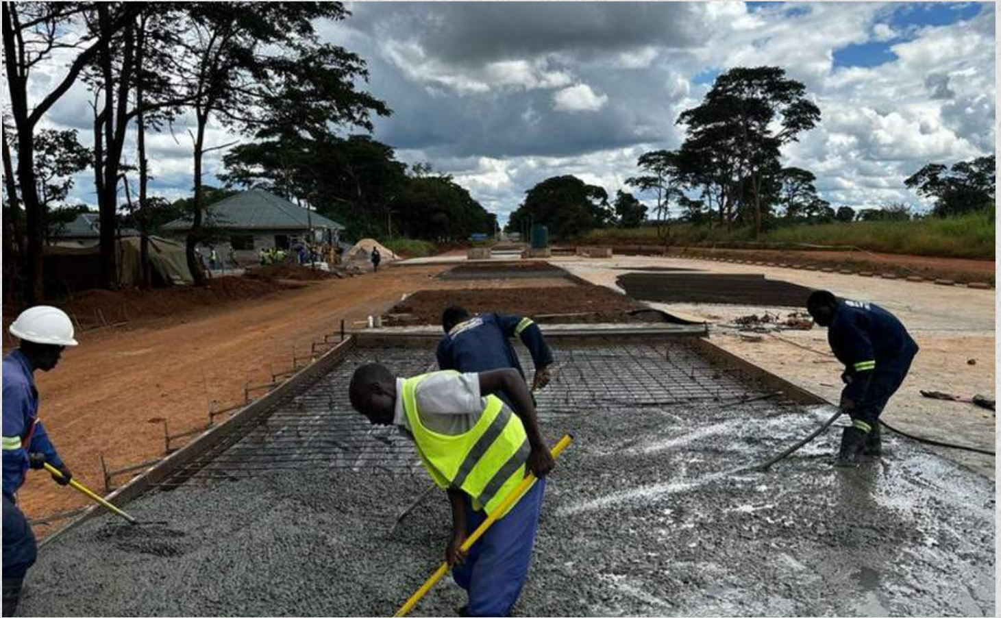
Works to upgrade the Mpongwe Toll Station from Class C to B located along the Luansobe-Mpongwe Road underway.
