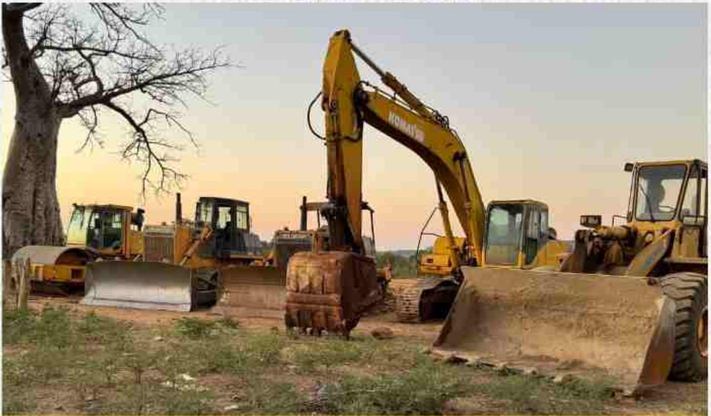
Site mobilization for rehabilitation works of the Batoka-Maamba Road in Southern Province.
