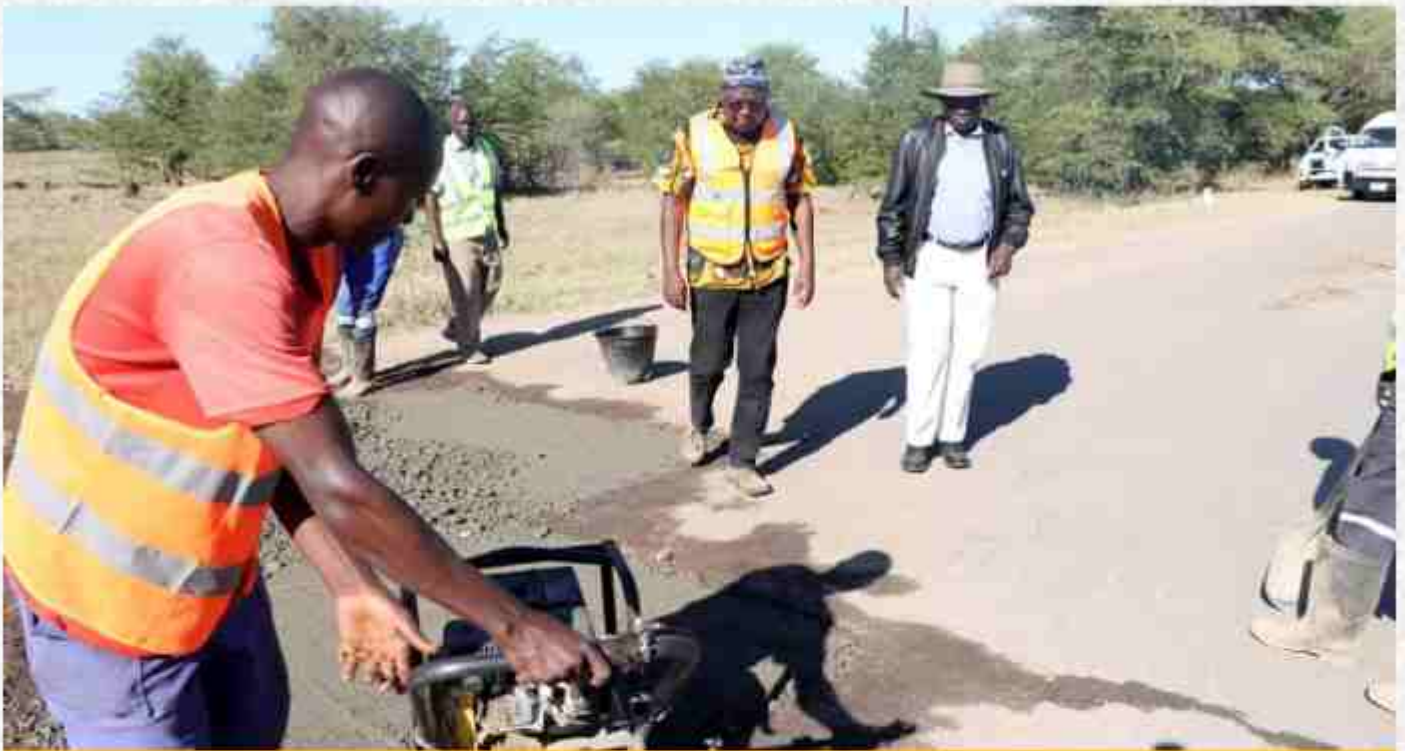
Infrastructure, Housing and Urban Development Minister, Hon. Eng. Charles Lubasi Milupi with the Southern Provincial Roads Engineer, Namalala Ghisala inspecting the ongoing holding maintenance works on the Kazungula-Sesheke Road.
