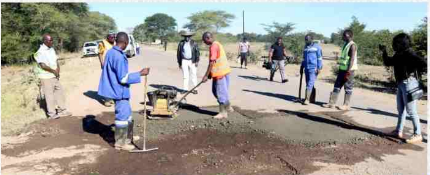
Infrastructure, Housing and Urban Development Minister, Hon. Eng. Charles Lubasi Milupi inspecting the ongoing holding maintenance works on the Kazungula-Sesheke Road.
