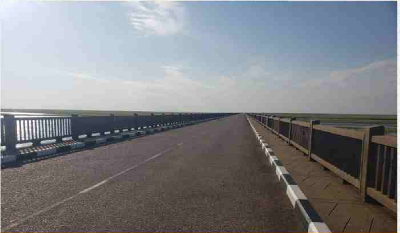
Painting works at Mukuku Bridge on the Tuta Road in Leapula Province.
